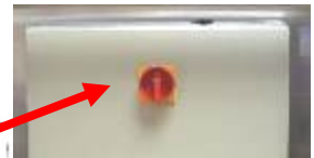
PROVER MAIN ISOLATOR
